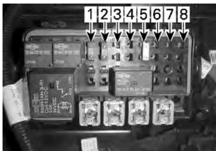
FUSES - RIGHT FUSE BOX
