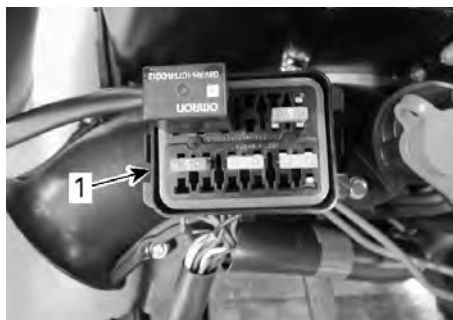
TYPICAL - FUSE BOX COVER REMOVED
