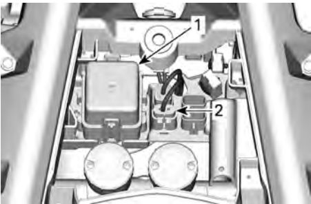
1. Front fuse box 2. DPS fuse
