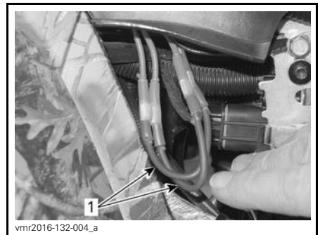
vmr2016-132-004_a 1. Fuse links
